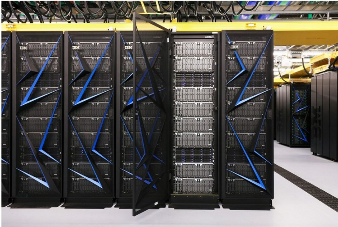
The IBM-built Summit supercomputer is the world's smartest and most powerful AI machine. Its racks are connected by over 185 miles of fiber-optic cables.
